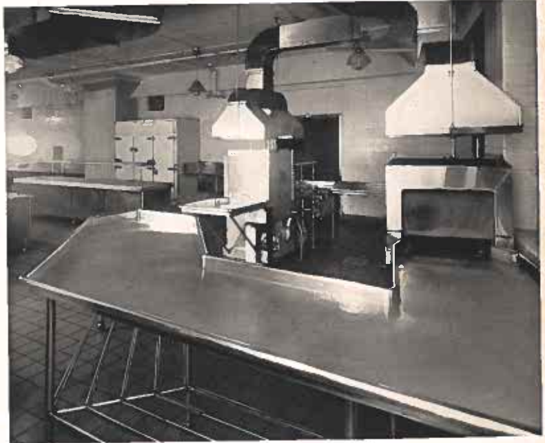
Dish Washing Equipment, Plate No. 923
