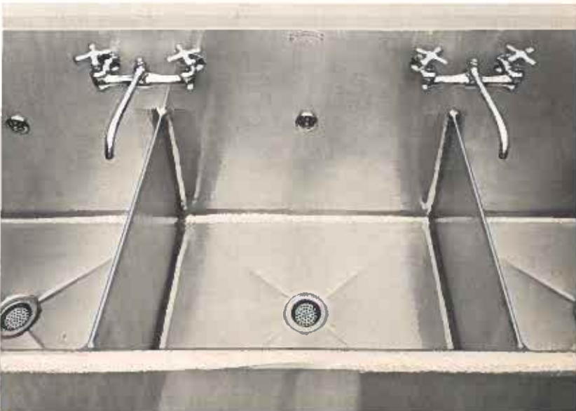
Close-up View of Sink, Main Kitchen, Plate No. 1512
