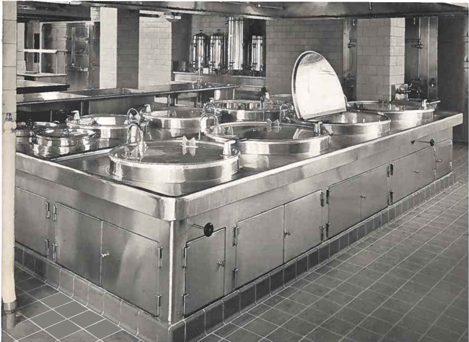
Kettle Enclosure, Main Kitchen, Plate No. 1507
