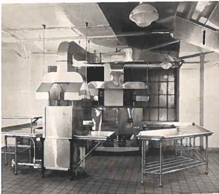
Dish Washing Equipment, Plate No. 926
