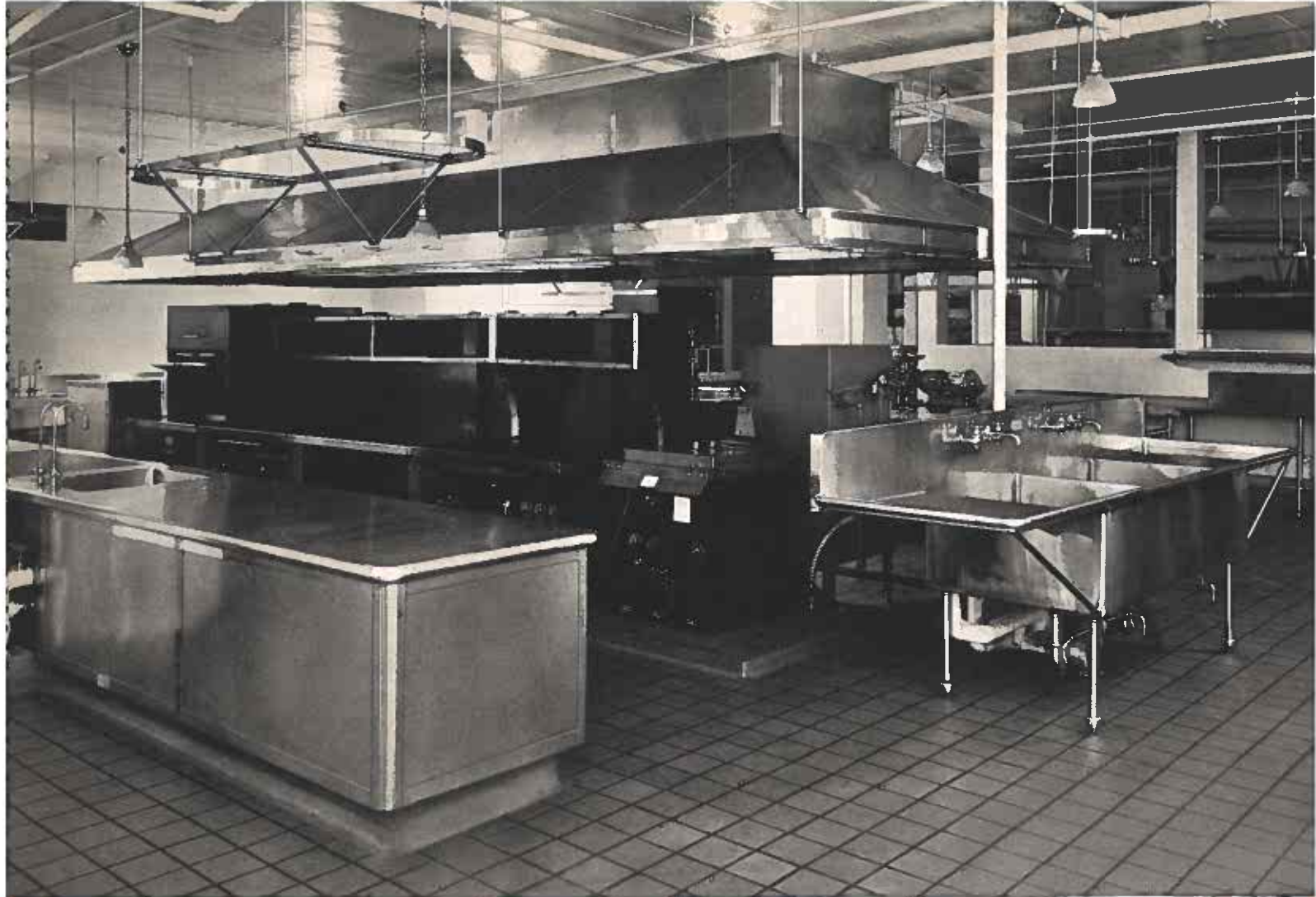
Main Kitchen, Plate No. 916
